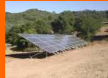
On Grid 6200 watt
